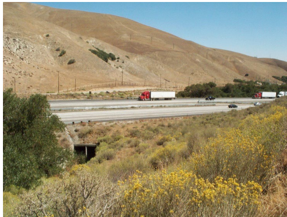
Culvert on Interstate-5 for Gorman Creek with Hungry Valley State Park in the foreground. Note steep degraded slopes on far side of I-5.
